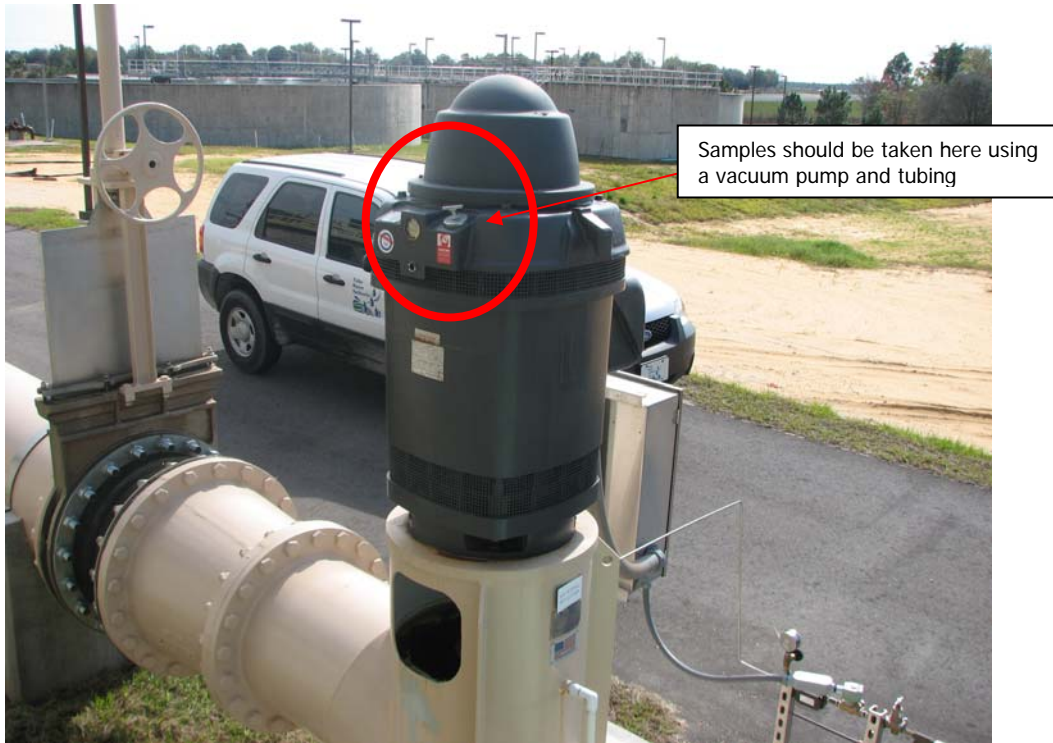
Internal Recycle Pump
